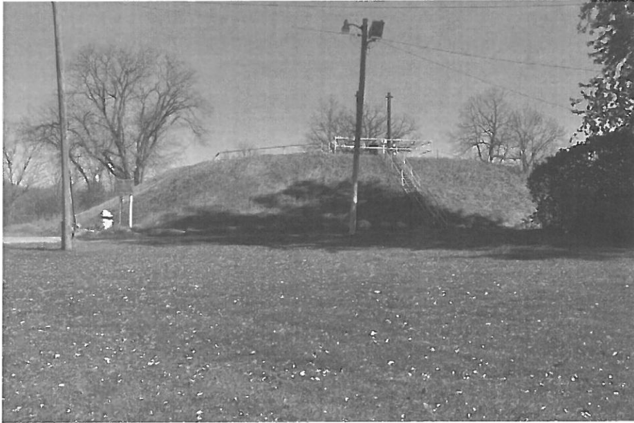
Fig. 126. OT-FRI-005. Taplin Gorge, embankment at southwestern end of canal with steel steps climbing it; penstock is buried under grass in foreground (facing E)
