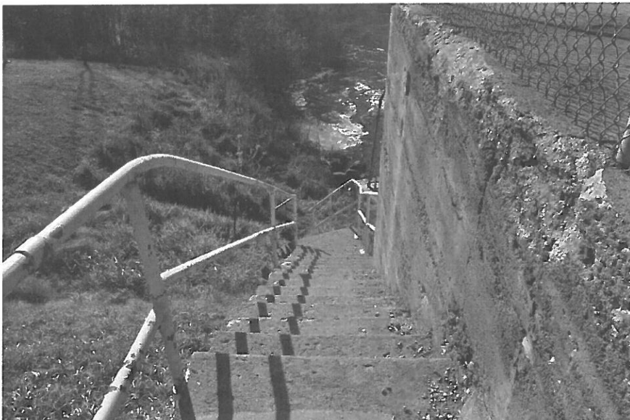
Fig. 105. OT-BUS-003. Pisgah Dam, concrete steps descending the southern side of the powerhouse (facing SW)
