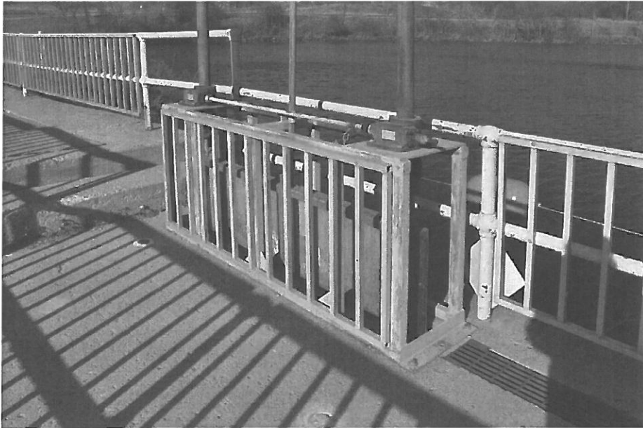
Fig. 100. OT-BUS-003. Pisgah Dam, spillway gate mechanism at top of spillway (facing N)
