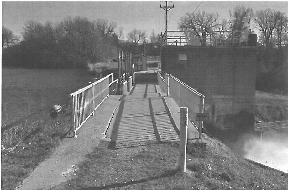
Fig. 98. OT-BUS-003. Pisgah Dam, northern end of spillway from embankment, concrete wing wall at lower left (facing SE)
