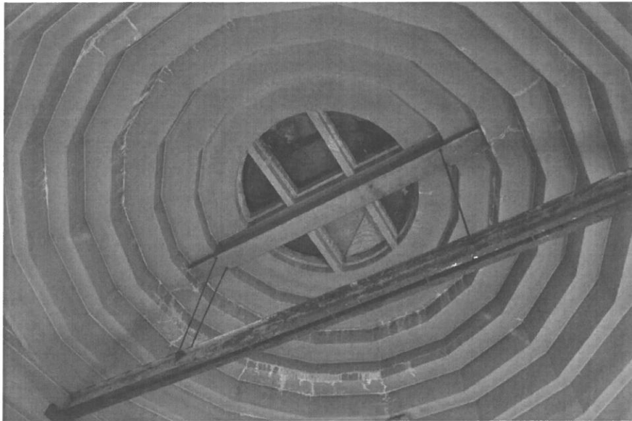
Fig. 133. OT-FRI-005. Taplin Gorge, poured concrete ceiling of upper level of powerhouse (skylight glass covered due to leaking) (facing W)
