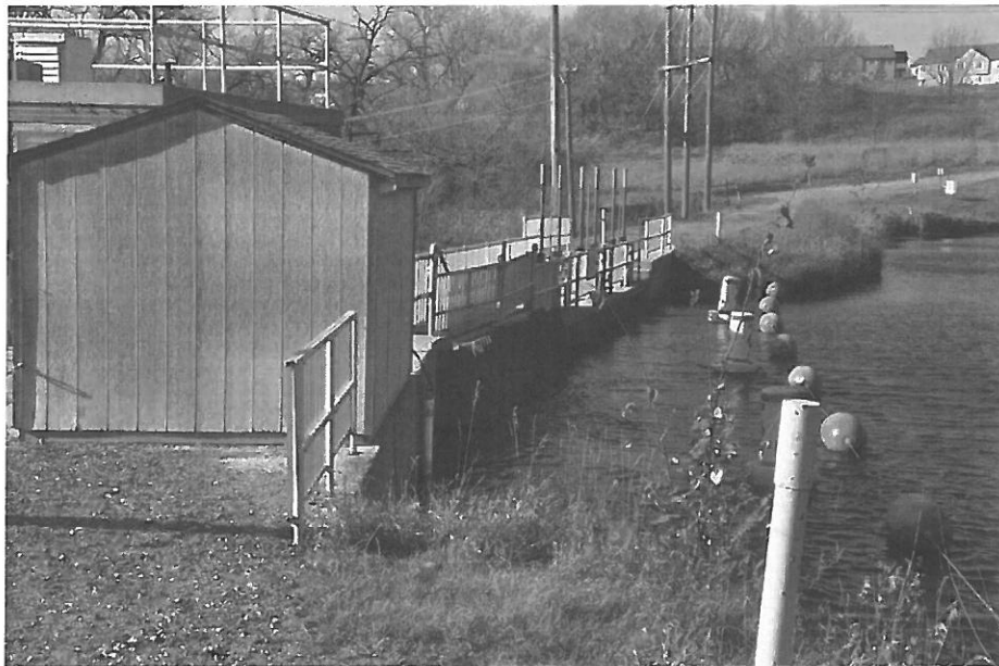
Fig. 95. OT-BUS-003. Pisgah Dam, reservoir and upstream side of the dam, modern stoplog shed at left; water enters the powerhouse just north (right) of the shed (facing NW)
