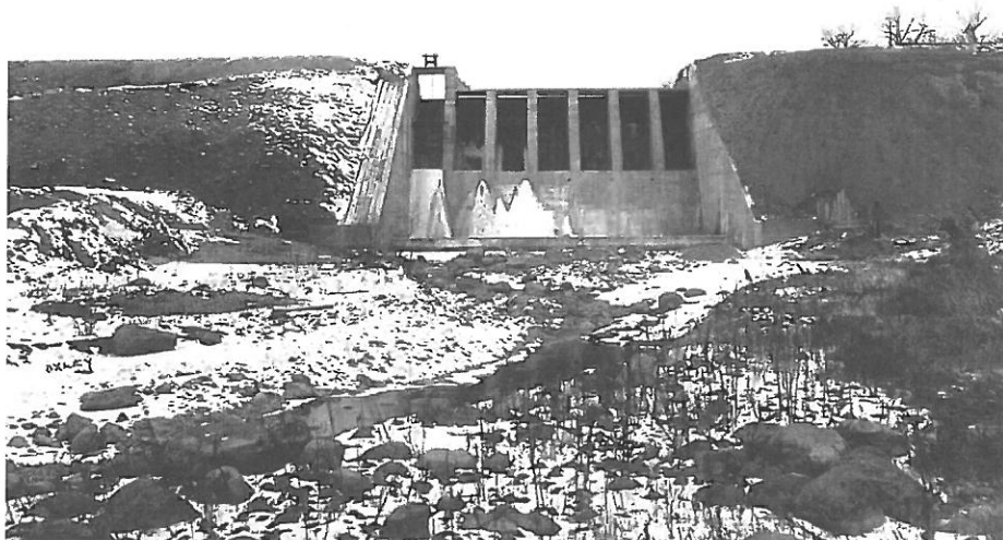
Fig. 110. OT-FRI-005. Taplin Gorge, southern side of dam; note fish ladder at left; 1926 photo by W. T. Oxley (Otter Tail Power Company Collection) (facing N)
