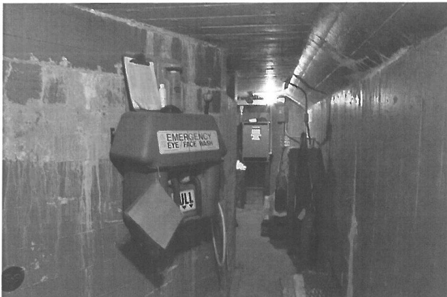
Fig. 136. OT-FRI-005. Taplin Gorge, lower level of powerhouse; at left is water-filled turbine chamber (facing W)
