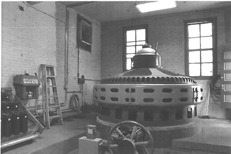
Fig. 101. OT-BUS-003. Pisgah Dam, generator and wicket gate mechanism, storage batteries at left, powerhouse entrance at right (facing NE)
