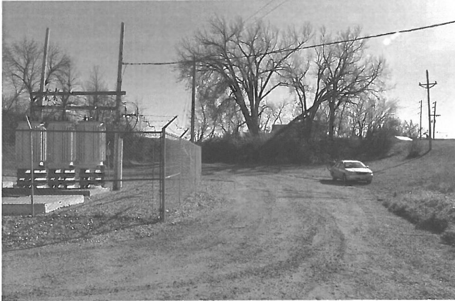
Fig. 92. OT-BUS-003. Pisgah Dam, service drive approaching from the south; substation and small parking area (facing S)
