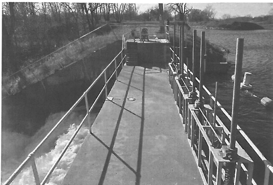
Fig. 117. OT-FRI-005. Taplin Gorge, walkway and gate controls on spillway; water is being diverted into the canal at upper right (facing W)
