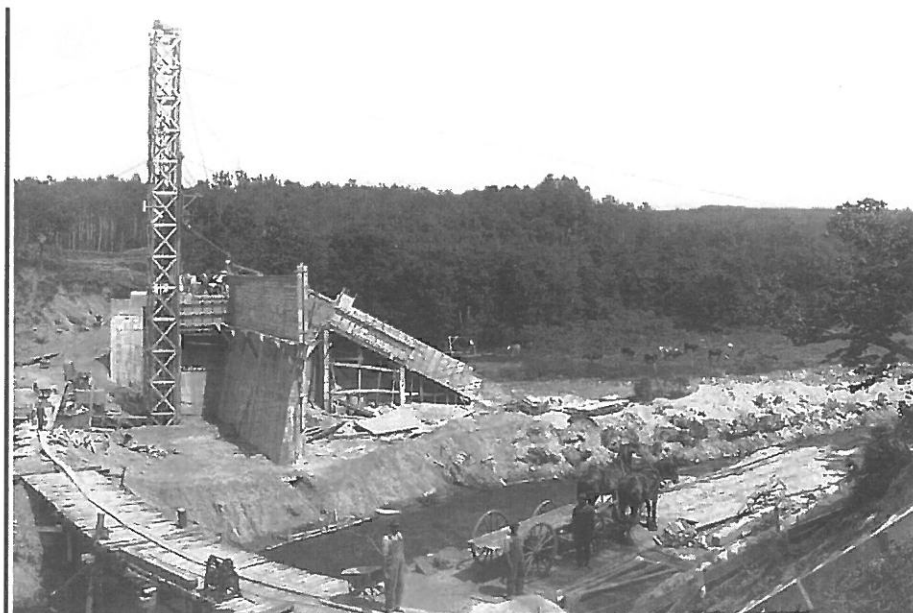
Fig. 107. OT-FRI-005. Taplin Gorge, dam being built, wooded eastern bank of river, 1925 photo by W. T. Oxley (Otter Tail Power Company Collection) (facing E)
