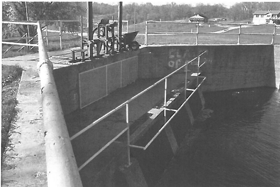
Fig. 125. OT-FRI-005. Taplin Gorge, penstock opening with three trash racks and gate mechanism (facing NW)
