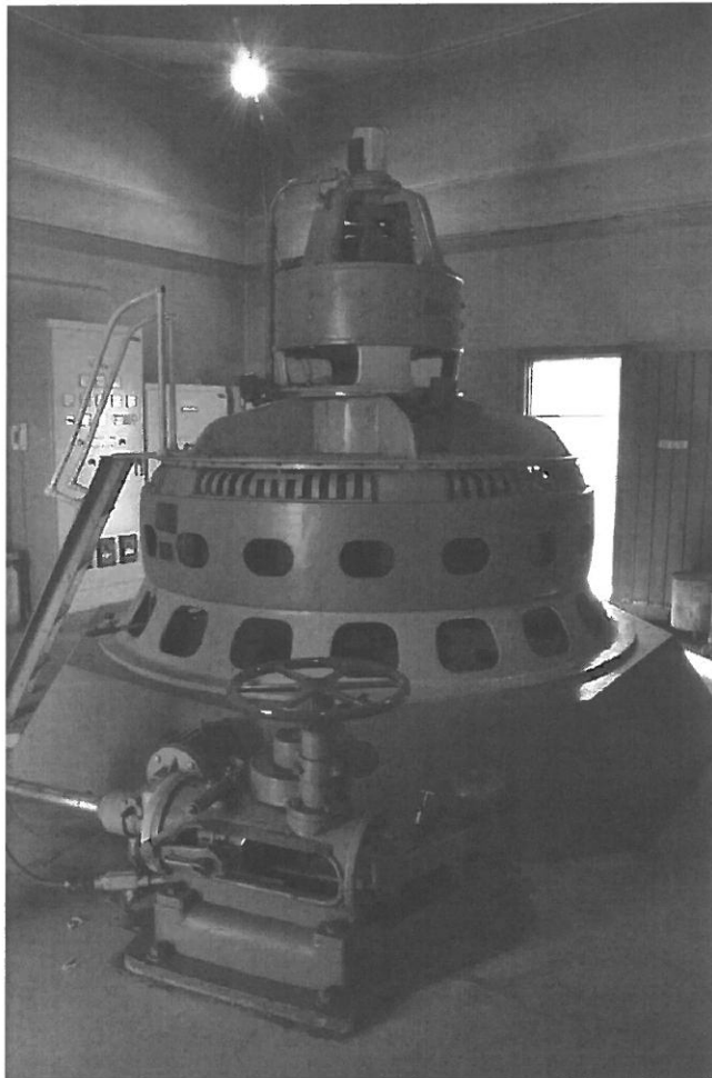
Fig. 132. OT-FRI-005. Taplin Gorge, 1925 Westinghouse generator, wicket gate gears and control mechanism in foreground (facing NE)
