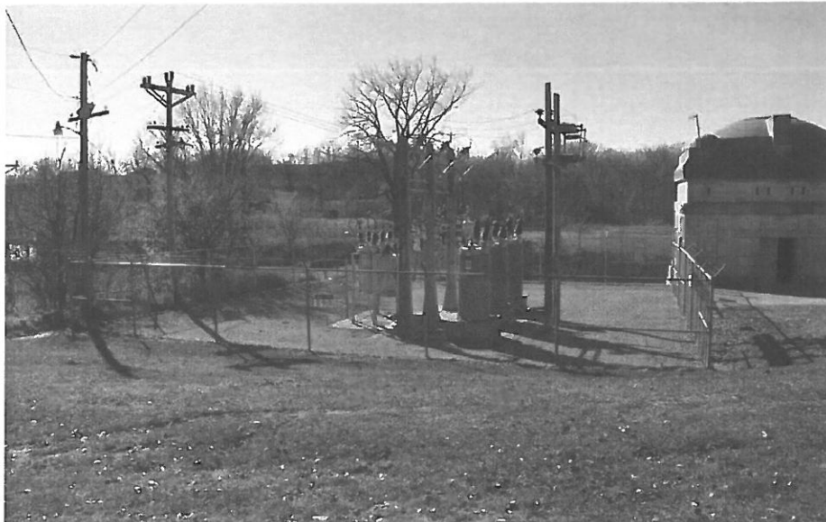
Fig. 127. OT-FRI-005. Taplin Gorge, substation (on original location) and powerhouse (facing W)
